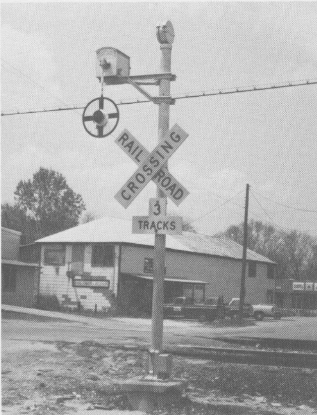
Figure 1- The wig-wag is essentially a motor driven banner equipped with a red light for night indication. These devices are obsolete and no longer recommended by the AAR.
